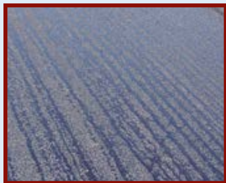
Poorly applied tack coat
